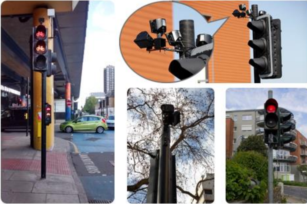
Figure 3 – Examples of signal equipment checked on a RARR walk – SCOOT detection, MVDs, IRDs, Pedestrian Cancel Detection, and faulty / damaged aspects.
