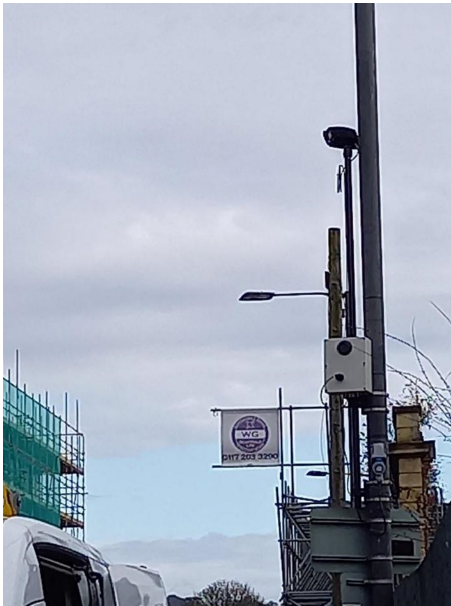
Figure 2 The installed Link and Detector
